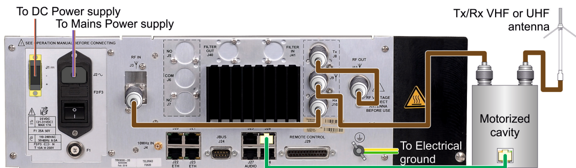
Figure 18 : One VHF or UHF antenna architecture with control of an external cavity
